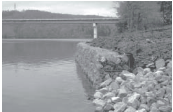
Gabions and Rock Riprap
